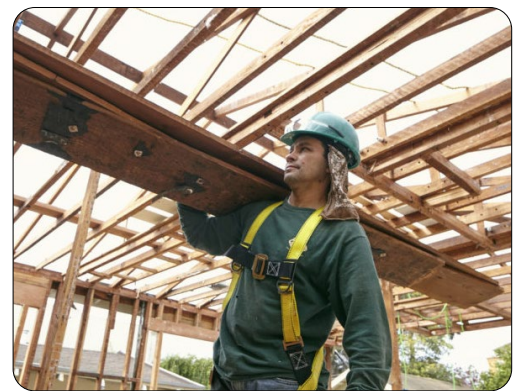
Salvaging wood from deconstructed buildings supports a growing movement to reuse valuable materials, reduce construction waste, and cut carbon emissions.
